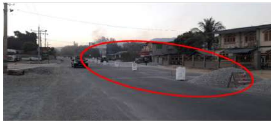
Road expansion and construction in Pyi Nyaung main roads. Open burning fire for asphalt.
